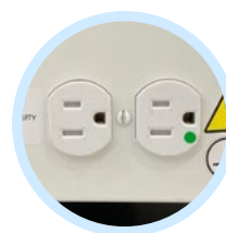
Hospital grade electrical receptacle
