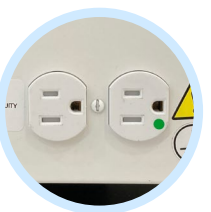
Hospital grade electrical receptacle
